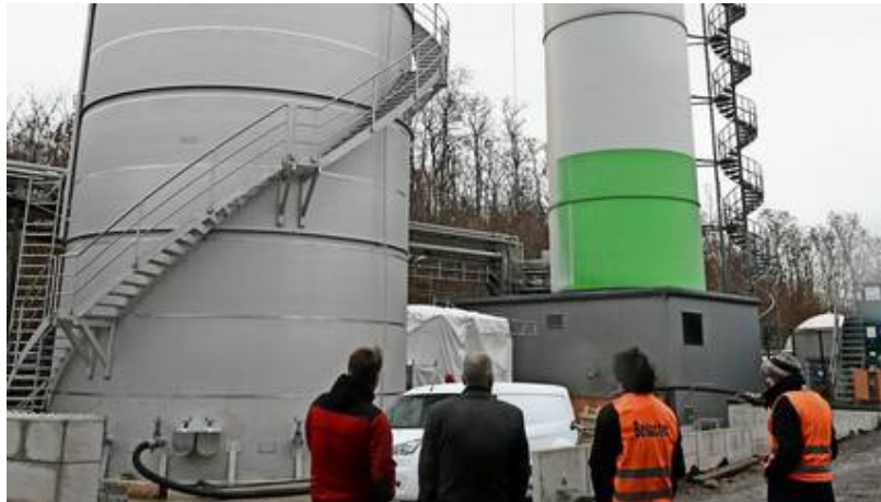
Figure 53: Anaerobic reactor at the Julius Schulte Trebsen paper mill.
