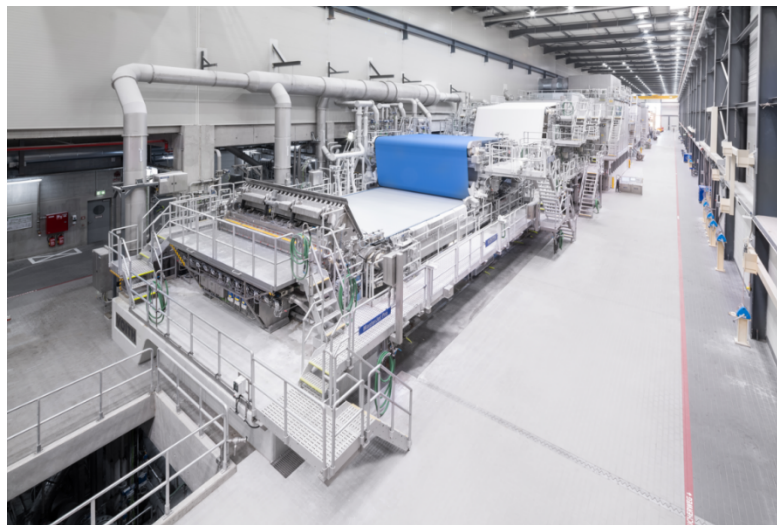
Figure 52: Production line 8 of the paper mill in Kehl.
